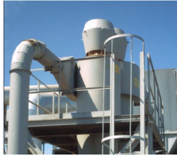
Fig.3. Source of 322 Hz frequency measured outside on the roof of production shop, with resonance of the cyclone construction.
