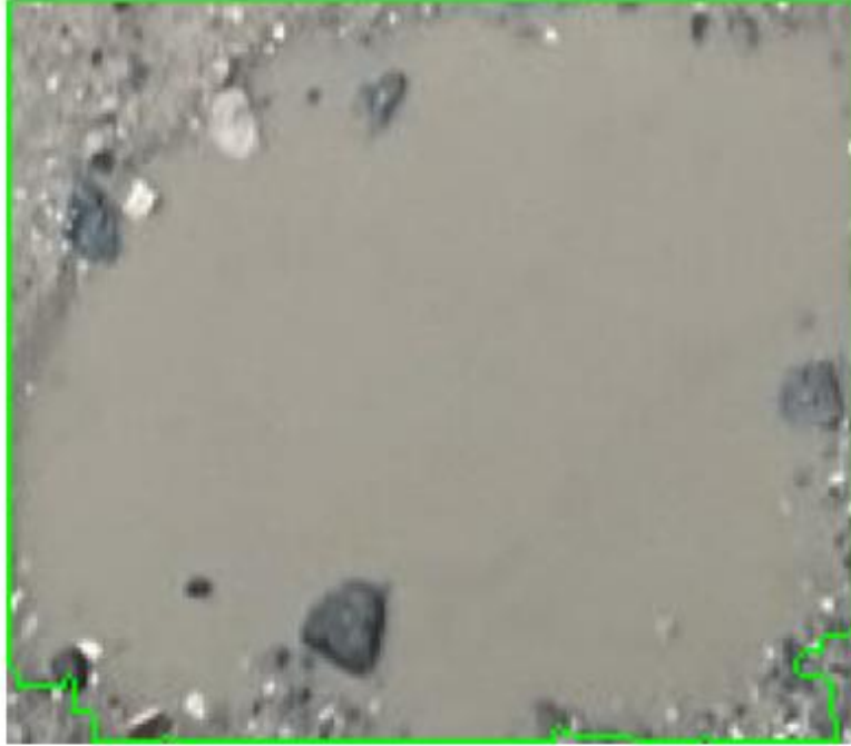
ROI 2 with Pothole Area Confidence: 0.86
