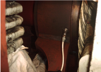
Fig.7 The 8 th bearing SPM2 transducer installed on the bearing housing inside generatortion
